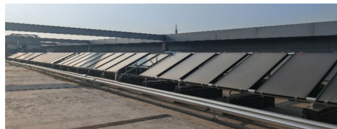
Thermal Energy Storage Facilities on Factory Roof
